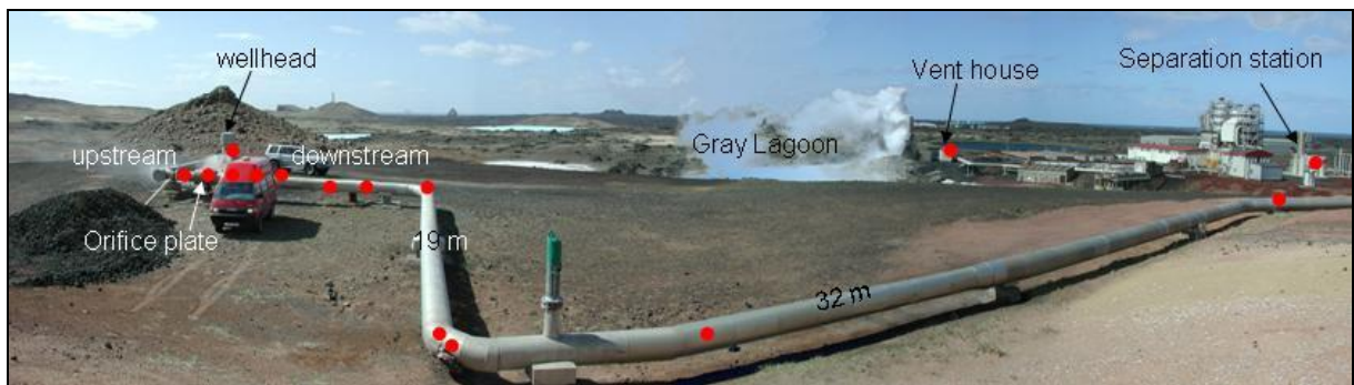
Figure 3. The pipeline from well RN9, Reykjanes geothermal field. Red dots show the location of samples mostly collected in the year 2000 (photo G. Ó. Fridleifsson).
