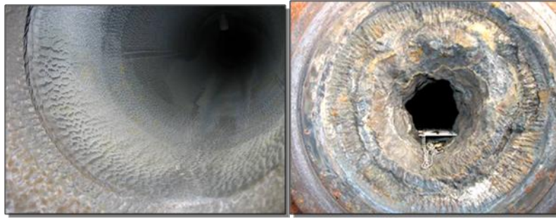
Figure 5. Photographs of surface pipelines looking upstream from the orifice plate (upper left); scales on the fluid flow control valve (14 cm long; upper right); and looking at scales downstream of the orifice plate medium-pressure well (lower left) and high-pressure wells (lower right). The pipeline diameter is 400 mm.
